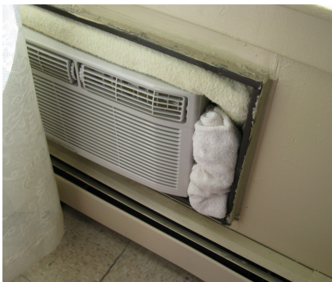
Fig. 7: Window AC installed in a sleeve
