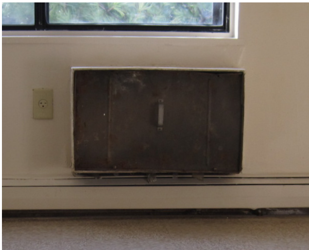
Fig. 5: Sleeve with metal cover instead of AC installed
