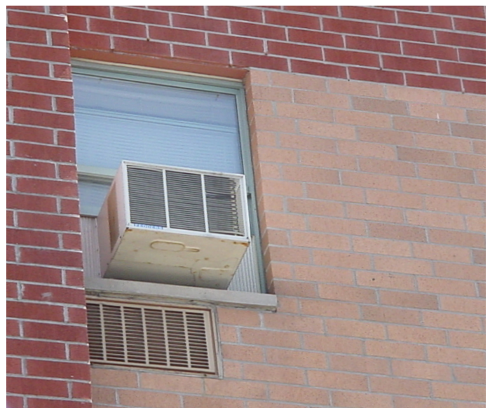
Fig. 8: Window AC above sleeve
