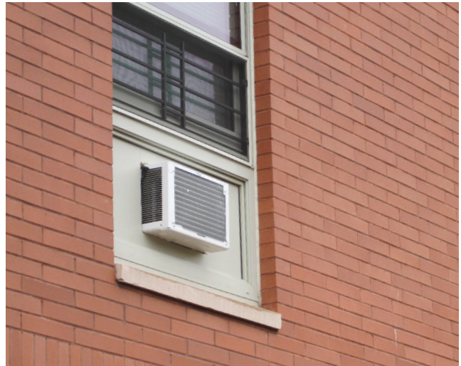
Fig. 14: Window AC installed in fixed panel below traditional double-hung window
