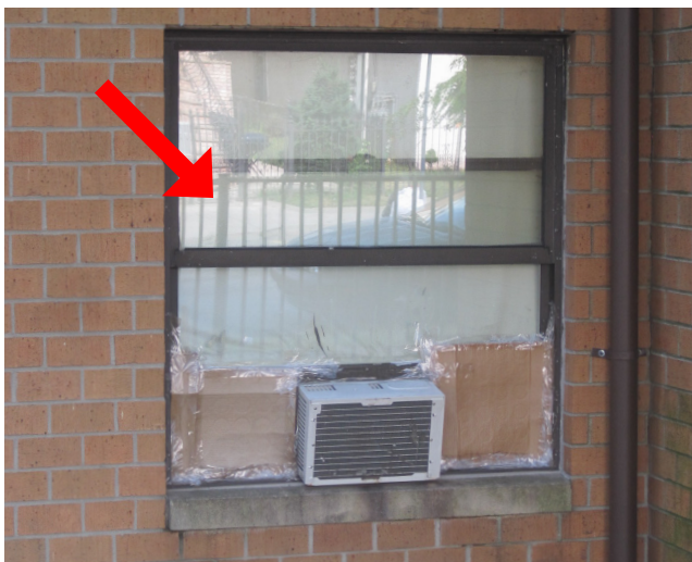
Fig. 3: Bad double-hung window installation
